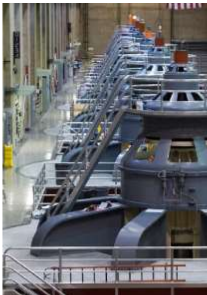
Figure 1. Lake Mead Generators Photo: Southern Nevada Water Authority
